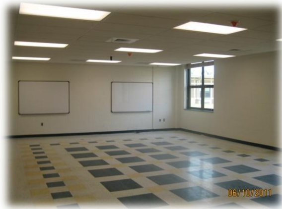
Figure 7: 2' x 4' Recessed Classroom Fixtures
